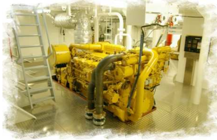
Figure 8 Engineroom mv Va Banque
